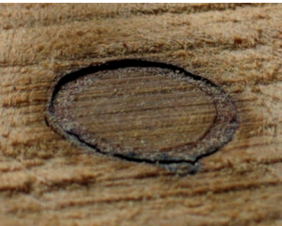
Pic.10 A dead knot that's a bit loose and needs to be checked in case it falls out. It is probably a candidate for replacement
